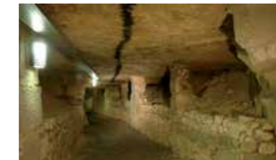
The "Workshop", a former quarry showing the two techniques for supporting the gallery roof used during mining operations for Lutetian limestone. © DAC / Christophe Fouin
